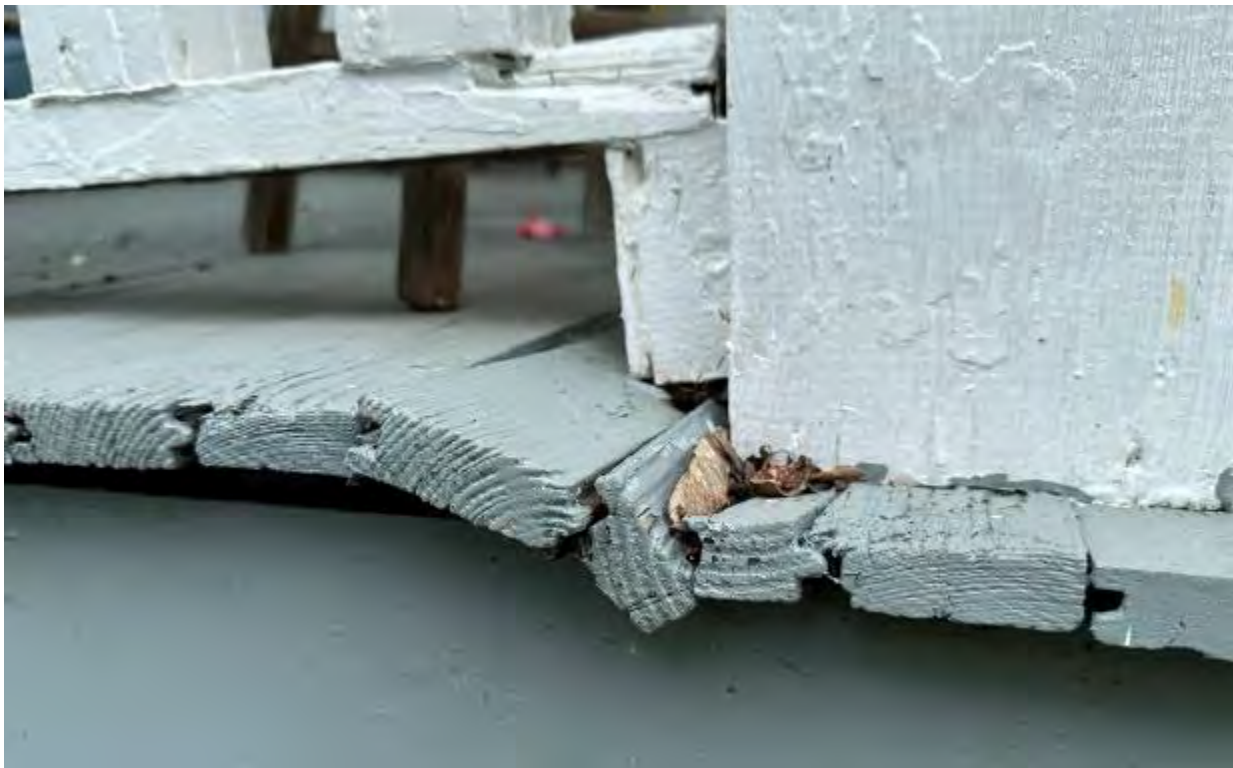
(Above) Evidence of deterioration.
