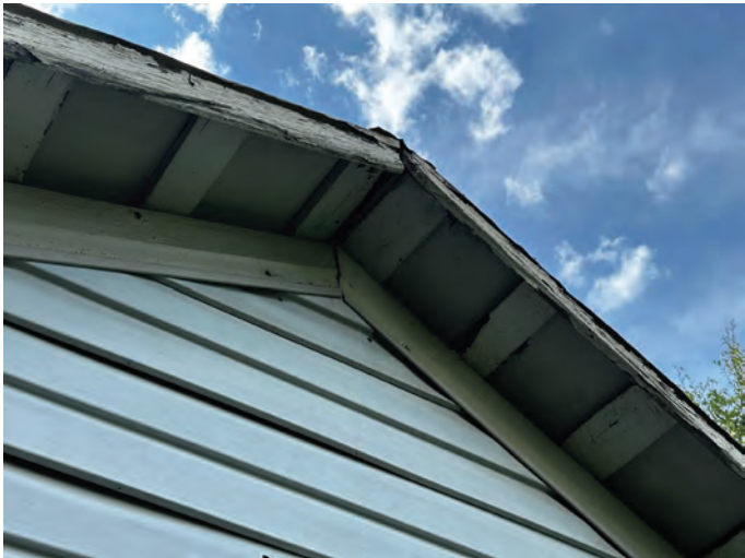
Exhibit A – Staff Photographs (Site Visit September 2023)
