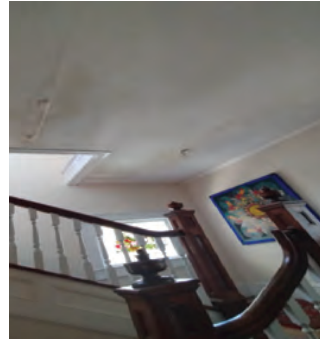
EXISTING WATER DAMAGED ENTRY ROOM CEILING AT FRONT OF HOUSE NO 6 Page 11
