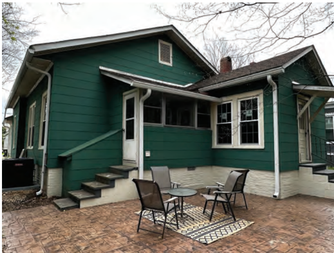
Figure 11 Window Detail (New Vinyl Replacement Windows). Site Visit 3-26-2024 by Kyle Harris, HPC Staff Liaison.
