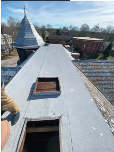
DESECRATED ROOF TILES NO 4
