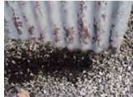
Corrosion of corrugated iron cladding is often the result of changes in ground level.
