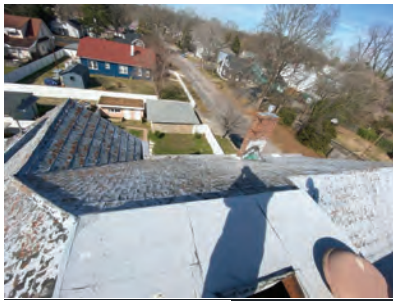
DESECRATED ROOF TILES NO 3
