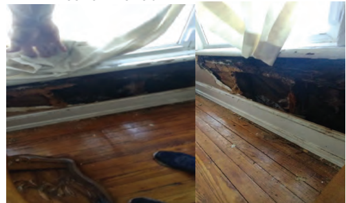
EXISTING WATER DAMAGED 2 ND FLR REAR BED ROOM NO 9 Page 13
