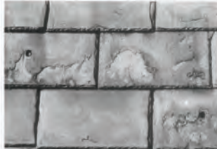
This detail shows slate delamination caused by a combination of weathering and pollution. In addition, the slates have eroded around the repair nails, incorrectly placed in the exposed surface of the slates. (Lower Ponahla Building, New Orleans, photo courtesy of Building Conservation Technology, Inc.)
