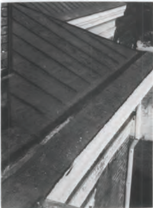
Repeated repair with asphalt, which cracks as it hardens, has created a blistered surface on this sheet-metal roof and built-in gutter, which will retain water. Repairs could be made by carefully heating and scraping the surface clean, repairing the holes in the metal with a flexible mastic compound or a metal patch, and coating the surface with a fiber paint. (Houma County Courthouse, Kingston, Tennessee, photo courtesy of Building Conservation Technology, Inc.)
