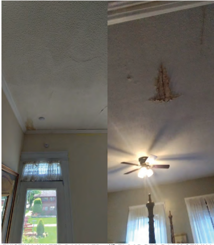
EXISTING WATER DAMAGED 2 ND FLOOR BED ROOM CEILING 1ST FLOOR 5 TH ST SIDE WALL AND NO 7
