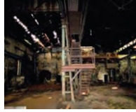
Part of a former historic iron works: notice the distinctive pattern of corrosion to the roof covering, which corresponds with the fixing points and sheet overlaps.
