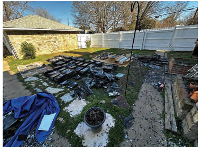
Figure 10 Site Visit 2-21-24 by Kyle Harris, HPC Liaison.
