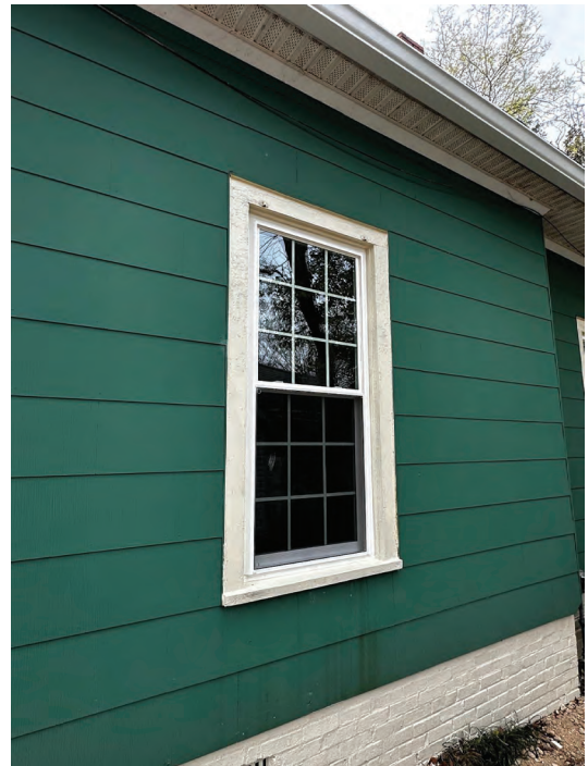
Figure 8 Window Detail (New Vinyl Replacement Windows). Site Visit 3-26-2024 by Kyle Harris, HPC Staff Liaison.
