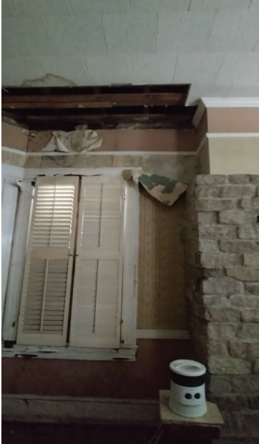
EXISTING WATER DAMAGED DINING ROOM WALL AND CEILING ON FIREPLACE WALL TOWARDS REAR OF HOUSE NO 2
