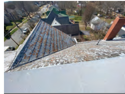
DESECRATED ROOF TILES NO 1.
