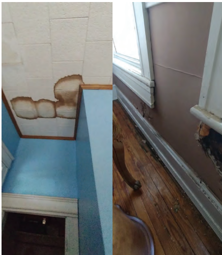
EXISTING WATER DAMAGED BEDROOM WALL CEILING AND FLOOR TOWARDS REAR OF BLDG. ABOVE DINING ROOM NO 10 Page 14
